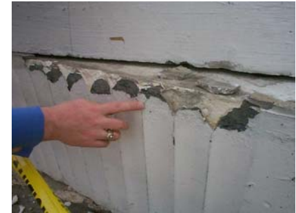
Detail of Damage Before Restoration
