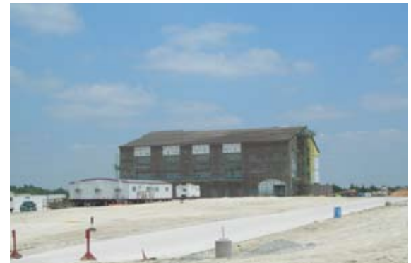
The new UNT Campus Master Plan provides for a build-out capacity of 25,000 students. The first building is under construction and scheduled to be opened in early 2007.
